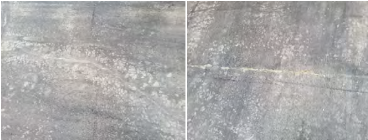
Photos of Cracks
