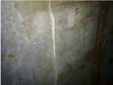
Photos of cracks
