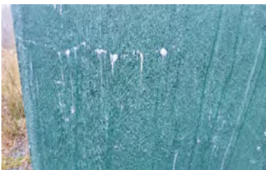
Photos of cracks
