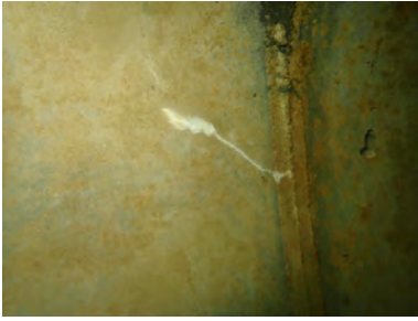
Photos of cracks
