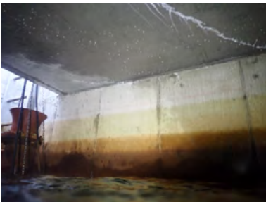
Photos of cracks
