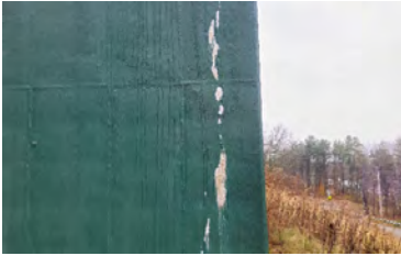
Photos of cracks
