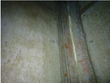
Photos of cracks
