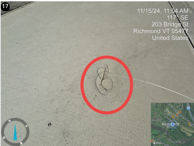
Large hole in the membrane.
