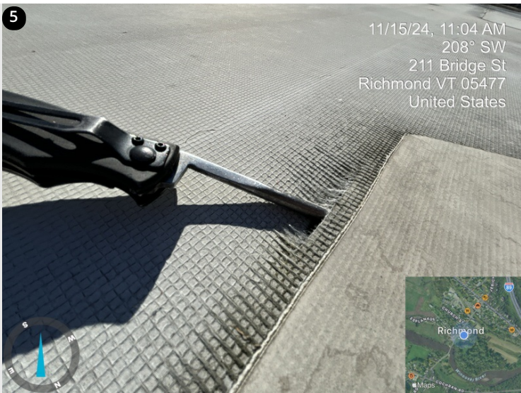
Hole through the degraded single-ply membrane. Exposed scrim throughout the membrane.
