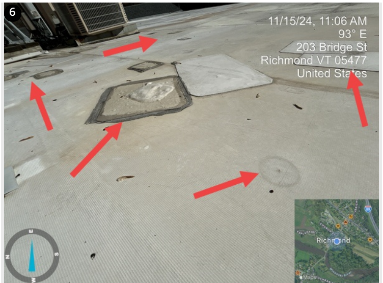
Fastener back out is prevalent throughout the roof sections. Several patches over the fasteners that have already punctured the membrane.
