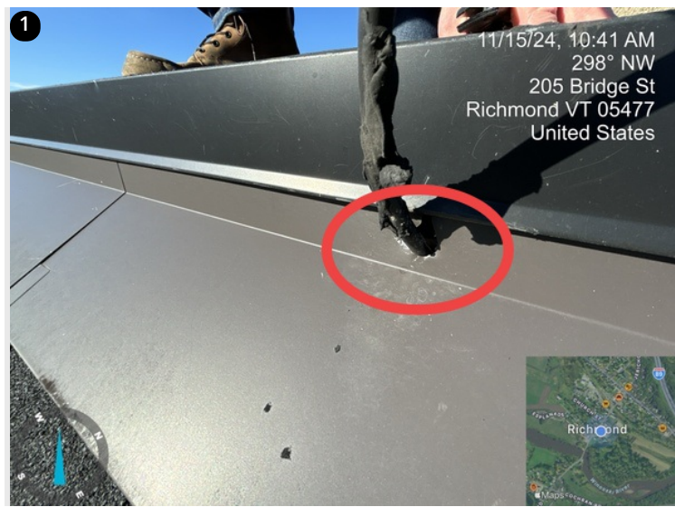
Improperly flashed penetration.
