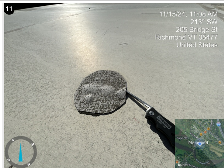
Failing previously installed patch. Incompatible materials (EPDM & TPO).
