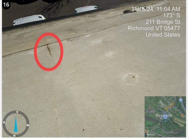
Cracked membrane due to degradation.
