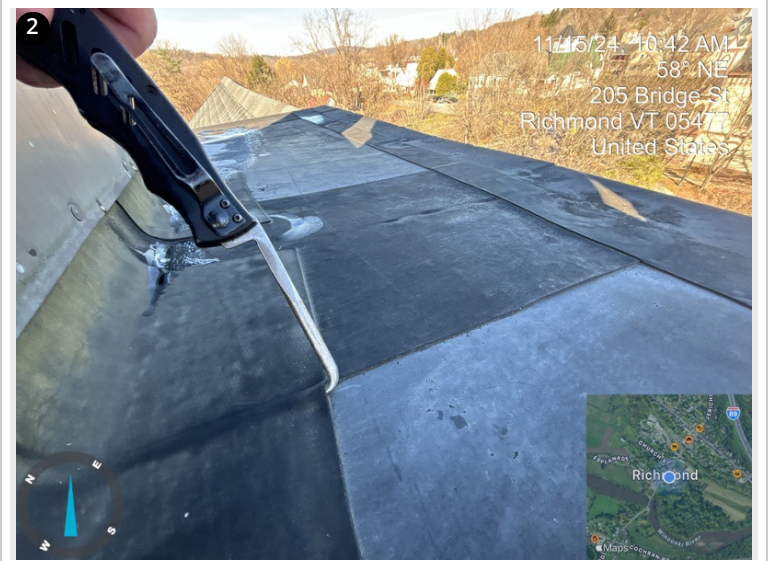
Open conditions surrounding flashing strips.
