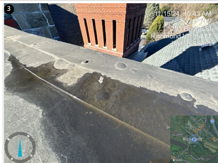
Minor ponding areas throughout the roof section. Perimeter flashing strip bubbling.
