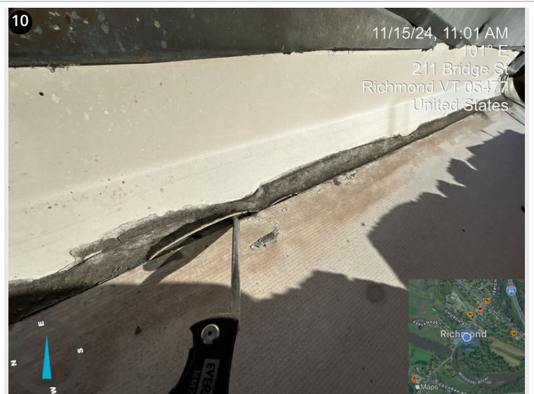
Perimeter flashings are deteriorated and cracked throughout.
