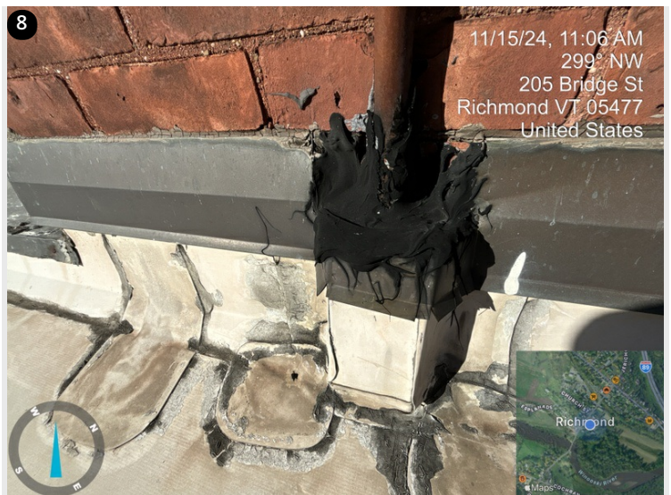
Improperly flashed penetration detail.
