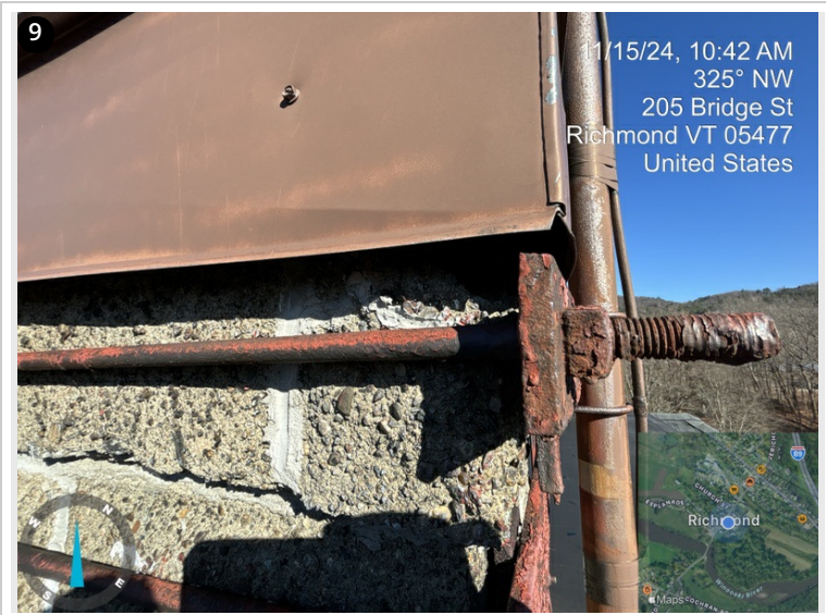
Deteriorated masonry throughout. Corrosion on the metal components attached to the chimney.
