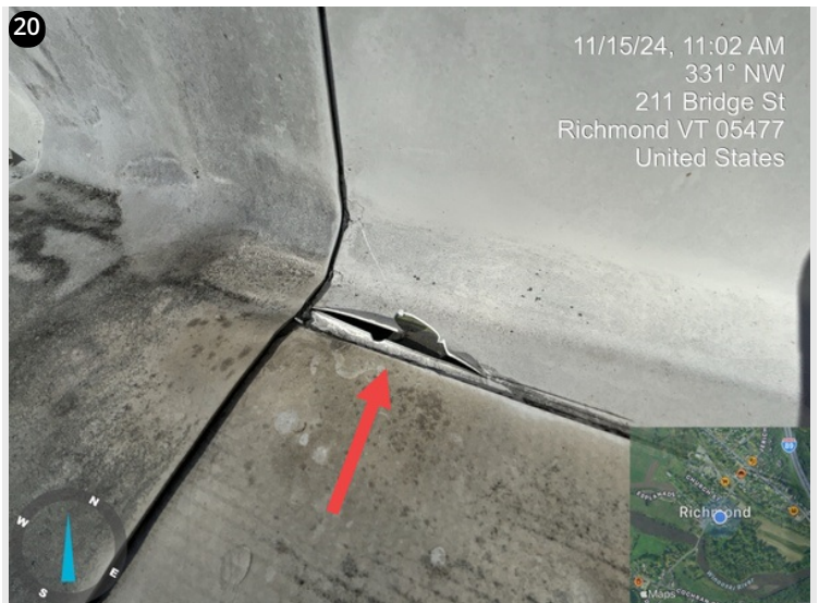
Failed flashing section. Membrane is brittle and is cracking and chipping away.
