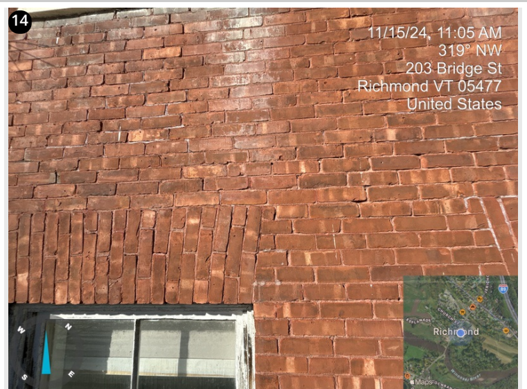
Masonry overview. Deterioration and degradation present throughout.
