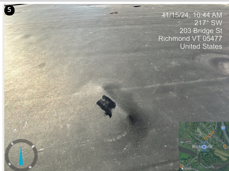
Fastener not fastened through the fastener plate.
