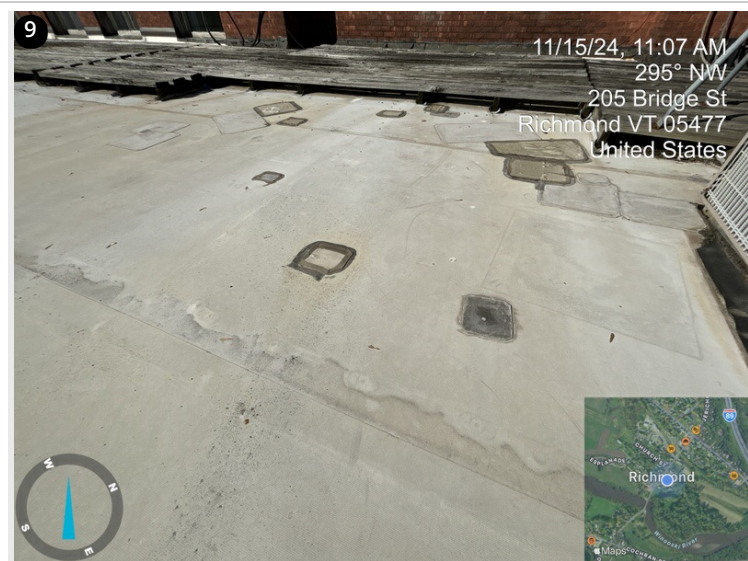
Several previously installed patches throughout the single ply roof system.
