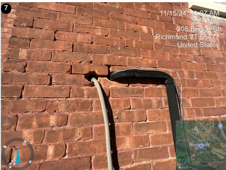
Improperly flashed penetrations in the masonry.
