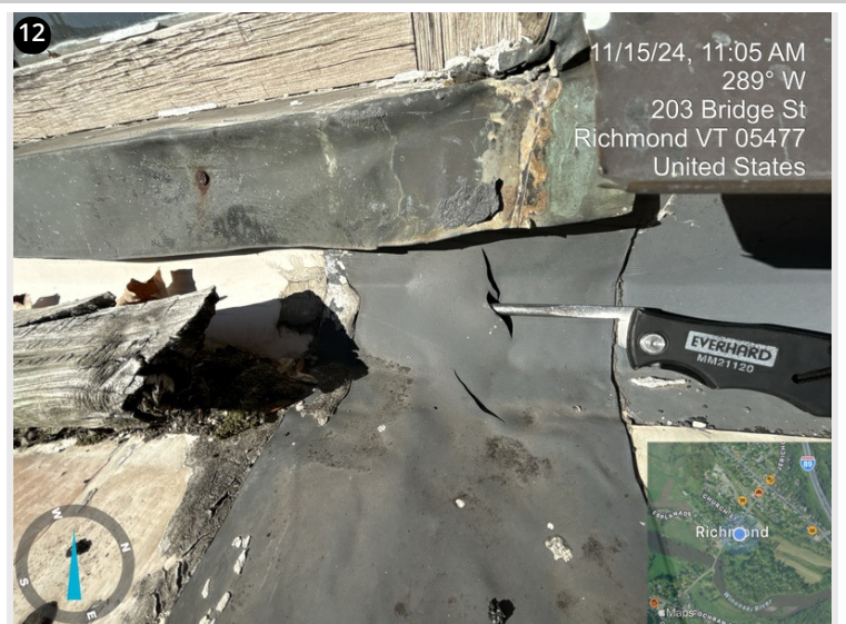
Degraded and split membrane.
