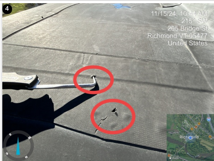
Punctures in the flashing strip.
