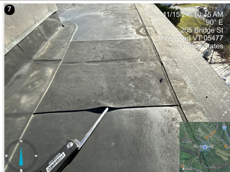
Flashing strip losing adhesion.
