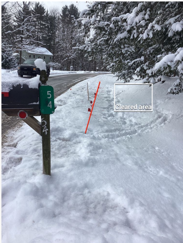
Point #3, Westall rd: electrical line crossing stake. Drill area should be moved back 3'-5'. Orange unmarked digsafe flag also present. Please refer to their report for findings.
