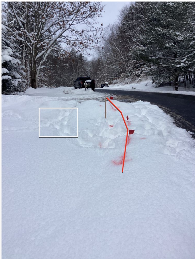
Point #6, Southview Dr: electrical line crossing stake. Drill area should be moved back 3'-5'. Orange unmarked digsafe flag also present. Please refer to their report for findings.
