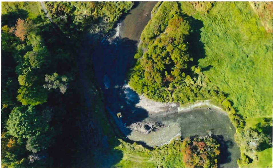
Clockwise from top left: Eroding bank along meander bend of Stevens River adjacent to private property and horse farm. The same meander bend following construction of bank stabilization measures. During the construction of stream bank stabilization measures along the Stevens River in 2018 we used a drone to inspect and document progress.
