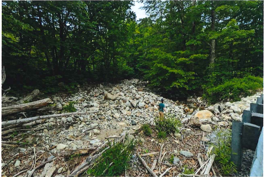
Initial visit to potential culvert upsizing project to be evaluated for HMGP funding. The stream crossing is located on Ball Mountain Brook, a steep tributary to the West River.
