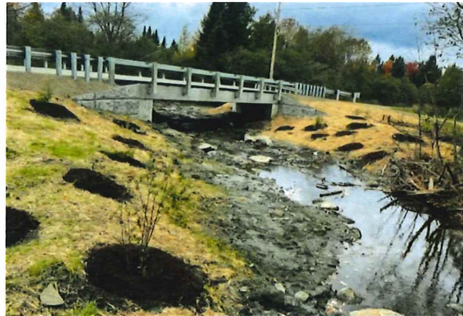
Precast footers, abutments, U-wall wingwalls, and precast concrete deck installation at Hutchins Farm Road.
