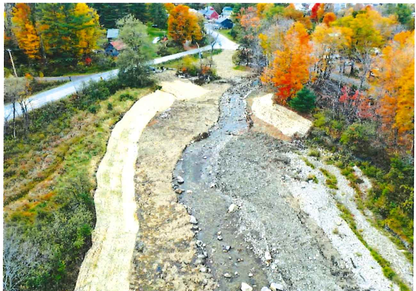
Aerial view of the Hands Mill Dam area collected in October 2024 following dam removal and restoration.
