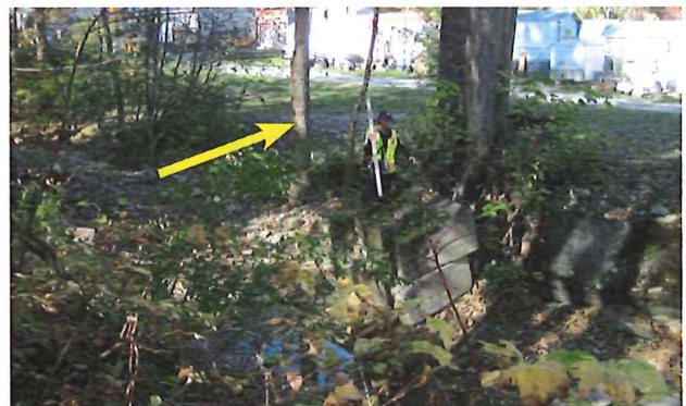
Yellow arrow shows where water has exited the channel upstream of old bridge abutments and concrete blocks (October 10, 2020)
