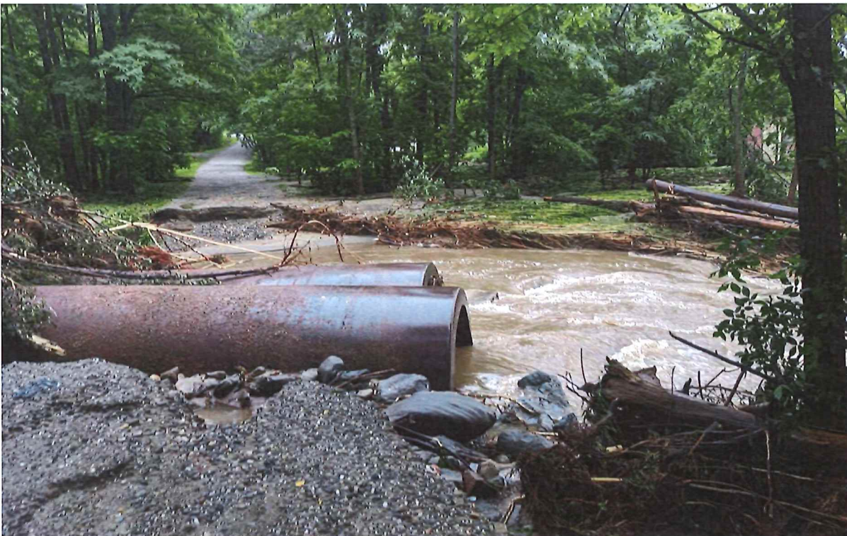
Figure 1: Washed out culverts on Snipe Island Brook under O'Neil Drive (photo by Jason McCune-Sanders)
